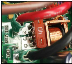
40 Amps fuse inside the controller
