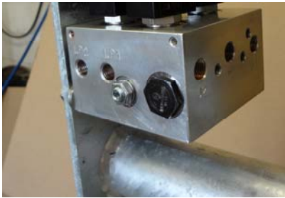
Manifold installation – front view.
